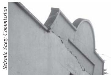
Figure 18 - Parapets. They are the tops of walls above the roof can fall off buildings like this one nearly did in Rio Dell during the 1992 Cape Mendocino Earthquake.
