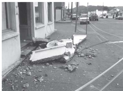
Figure 20 - Unbraced Parapets can Injure and Kill - This parapet on the front of the building in Figure 18 fell on the sidewalk.
