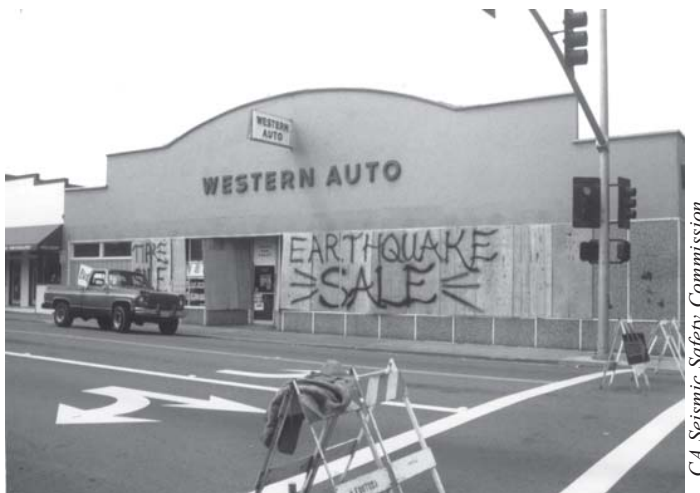
Figure 55 —The front window of this Fortuna auto parts store broke in the 1992 Cape Mendocino earthquake.
