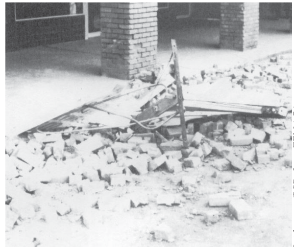
Figure 38 - The sign on this commercial building fell in the 1979 Imperial Earthquake.
