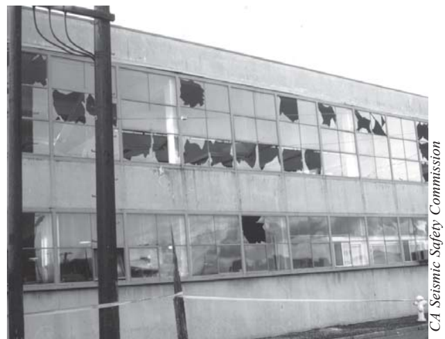
Figure 56 —The windows in this San Francisco building probably broke because its frame flexed too much in the Loma Prieta earthquake of 1989.
