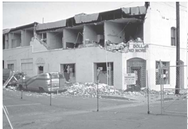
Figure 16 - The second-story wall of this unreinforced masonry building was not well-tied to the roof, and the building collapsed during the 1994 Northridge earthquake.
