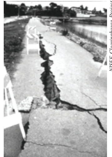
Figure 39 - Lateral Spreading. Loma Prieta Earthquake, October 17, 1989. Lateral spreading damage levee road along the San Lorenzo River.
