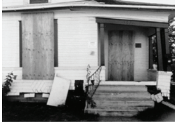
Figure 13 - This home wasn't bolted and slid off its foundation. Sometimes the damage can be so bad that houses have to be demolished.
