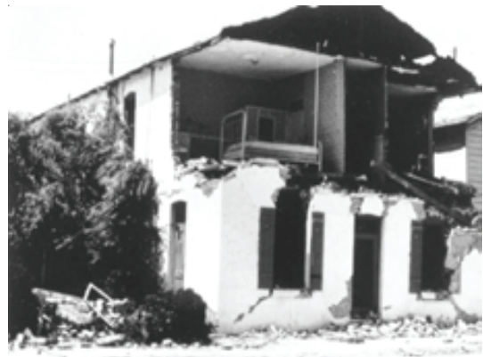
Figure 25 - The plaster-covered brick walls of this building collapsed during a recent earthquake.
