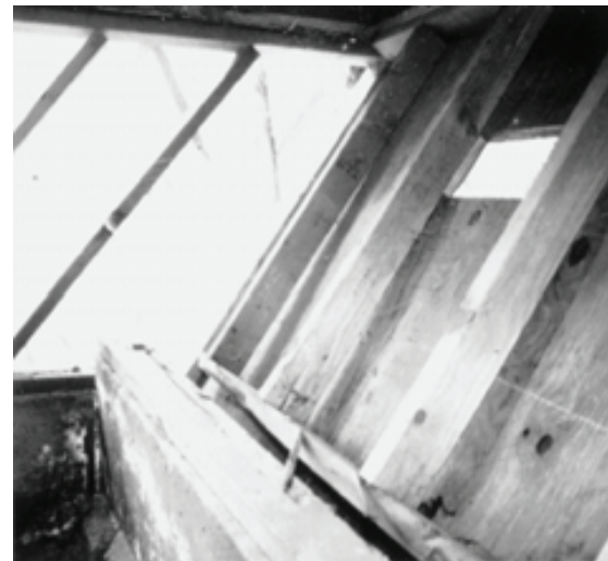
Figure 23 - This photograph shows an interior detail of a home similar to the one above, showing substantial damage to a building with an unbraced tall wall.
